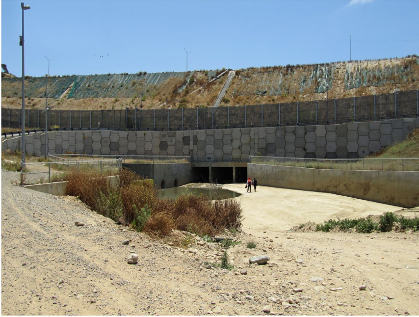
Figure 2. Los Laureles Creek drain culvert in the US–Mexican border fence near the Tijuana River estuary. Photograph by Peter Mörtenböck and Helge Mooshammer, 2011.
