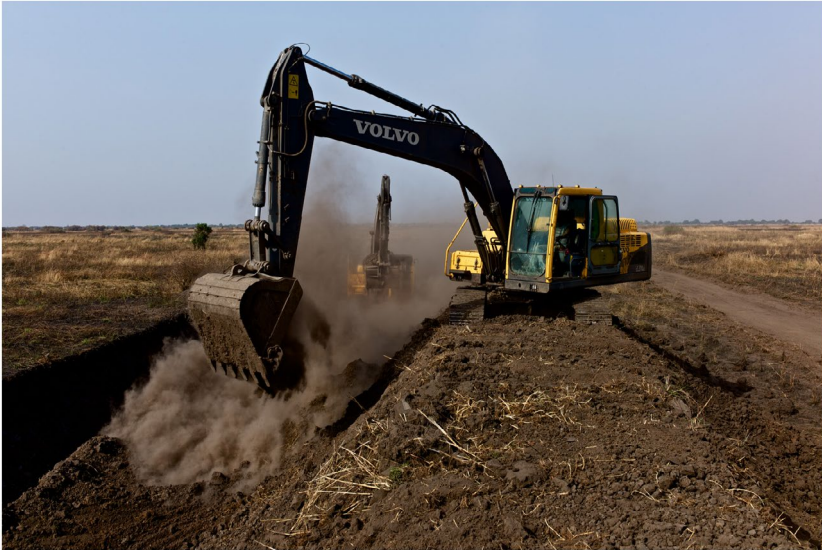
Figure 5. Building water channels for irrigation on the 100,000 hectare farm of indian investor Ram Karuturi in Gambela, Ethiopia. The Farm , 2012, part of the ongoing research project LandRush by Frauke Huber and Uwe H. Martin.
