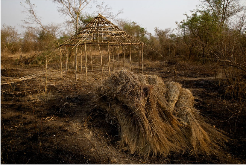
Figure 4. Construction of resettlement houses in Ibago, Ethiopia. The Farm , 2012, part of the ongoing research project LandRush by Frauke Huber and Uwe H. Martin.
